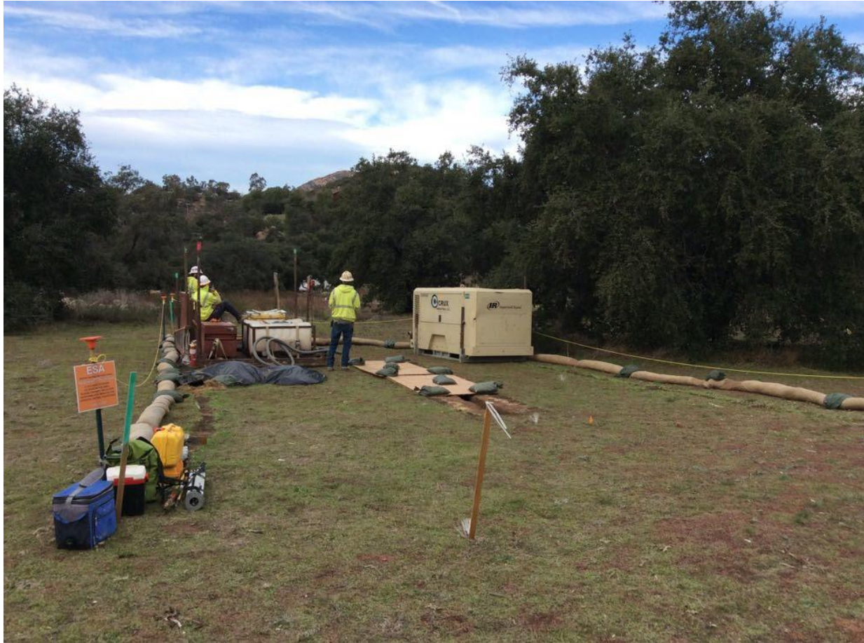
Photo 3: At a site along TL 625C that occurs within or adjacent to an archaeological or cultural resource site, the cultural ESA was clearly delineated and avoided by construction crews in accordance with the HPMP and APM CUL-03.
