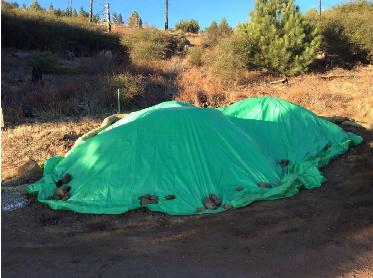
Photo 6: A spoils stockpile near Station 60+00 (C 79A) was covered with plastic sheeting to prevent erosion in accordance with the Erosion Control Plan and SWPPP.
