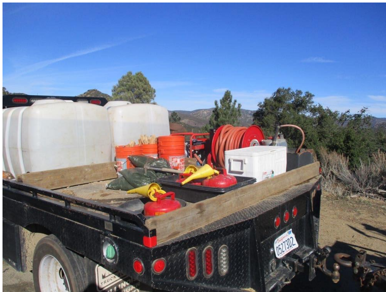
Photo 5: To prevent leaks and spills from being discharged into the soil, fuel canisters at Pole Z774863 (TL 6923) were staged within drip pans in accordance with MM PHS-2 and the SRNP.
